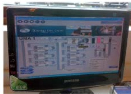
Building climate control system
